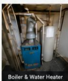
Boiler & Water Heater
